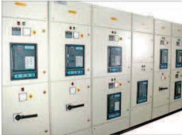
LT Distribution Panels/PLC Panels /Control & Relay Panels
